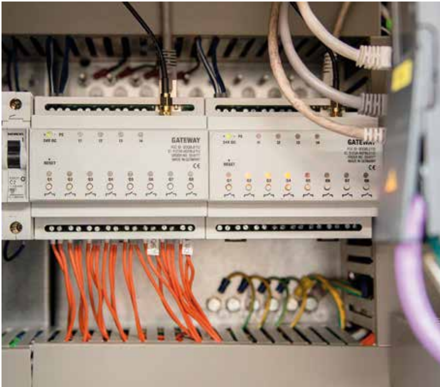
Gateway, verbaut in Schaltschrank Gateway, installed in control cabinet
